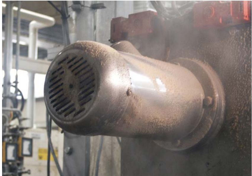
Above. Lafert 'Marlin' stainless steel motor in the working environment at Weetabix.
